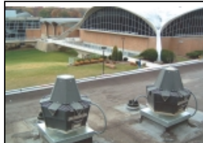
Tjernlund Specified Systems were used in four buildings on the university campus. Shown are two Auto-Draft® rooftop mounted inducers.
